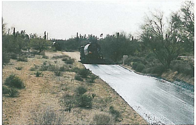
BST treatment - An ISS paving crew covers a dirt road in a rural Phoenix neighborhood.
